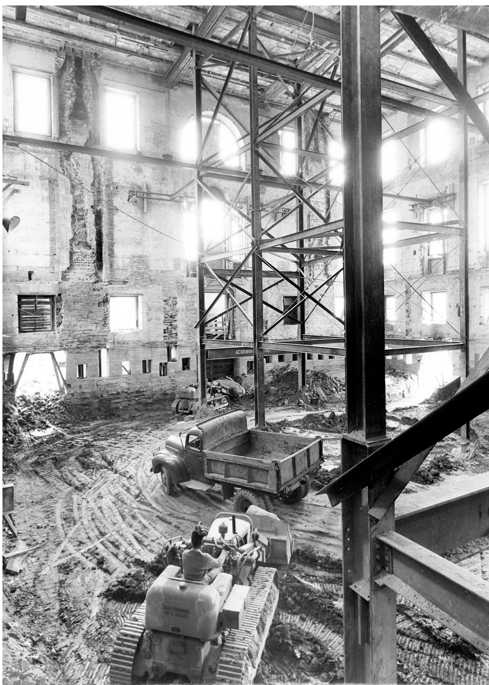
Harry Truman's renovations to the White House served as perfect cover to bury a new bomb shelter under the north lawn.
