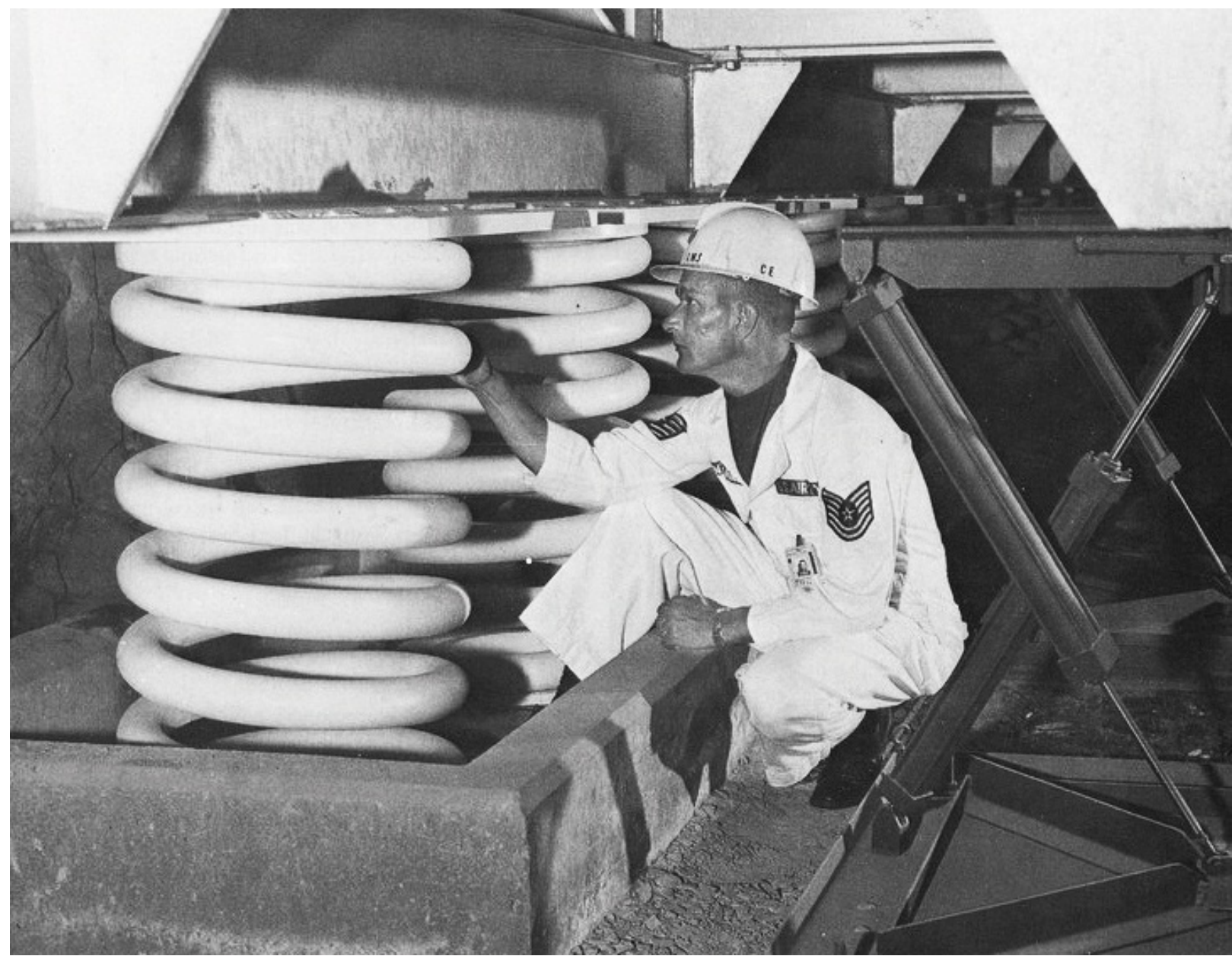
The buildings inside the mountain were mounted on man-sized springs to sway during a nearby blast.
