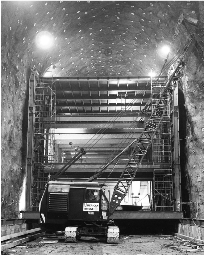
Inside the massive hollowed-out caverns, engineers built free-standing three-story buildings that would be the heart of NORAD.
