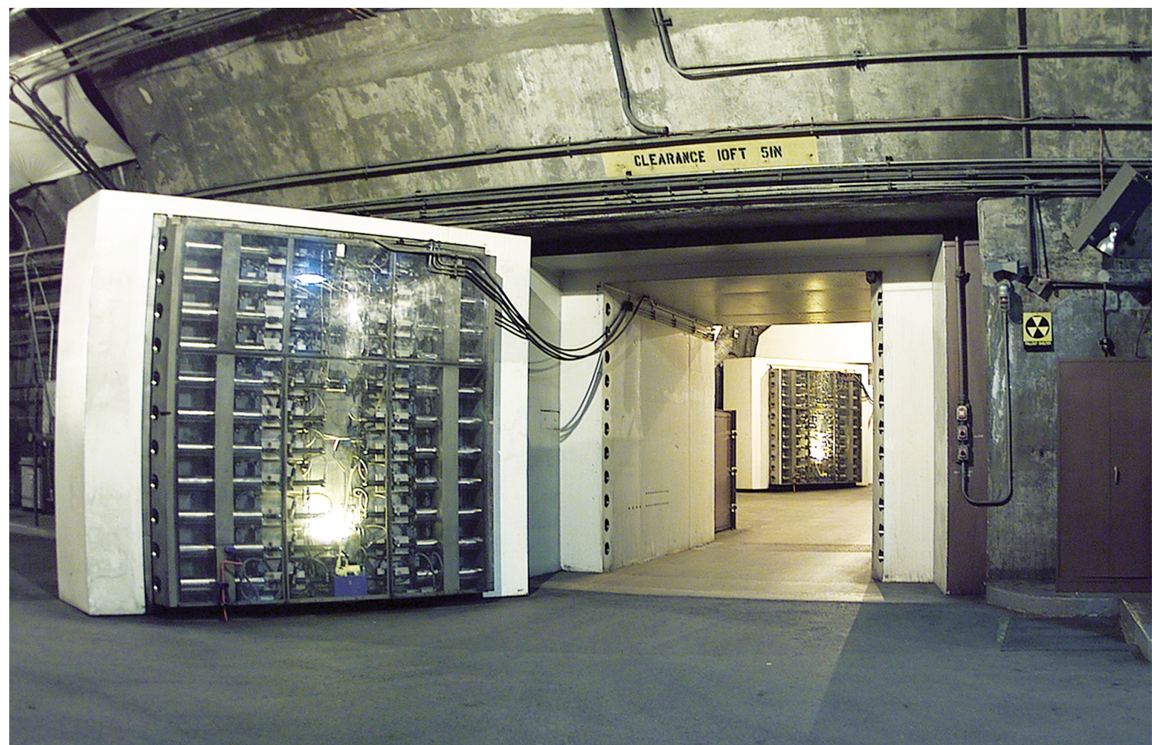
Deep inside the tunnels, massive blast doors could have sealed commanders away from an attack.
